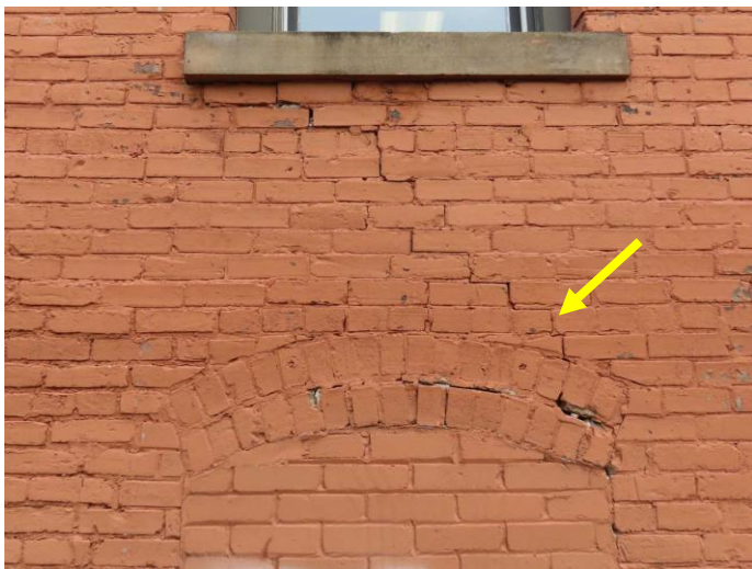
Masonry Cracking, Typical
