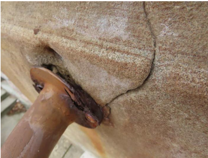
North Elevation Steel Handrail Attachment at Stone – Corrosion of the flanges and anchors is severe and causing damage to the adjacent stone.
