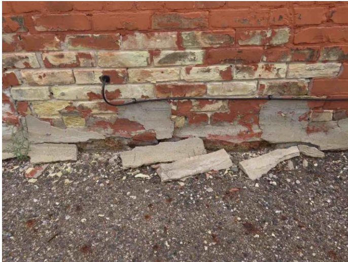
Severe Masonry Deterioration, Typical
