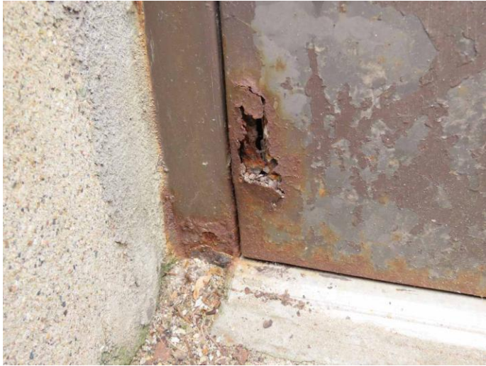
North Elevation Basement Door and Frame Corrosion
