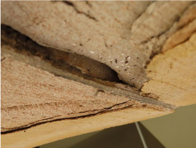
Stone Arch Delamination, Typical
