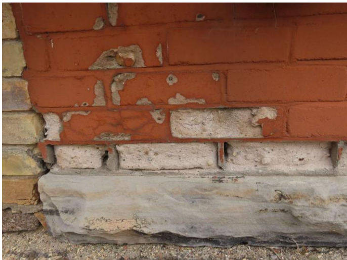
Severe Masonry Deterioration at Window Infill
