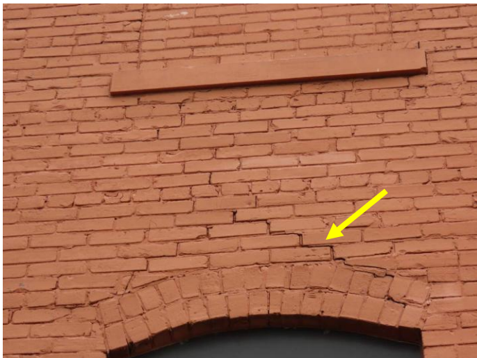
Masonry Cracking, Typical
