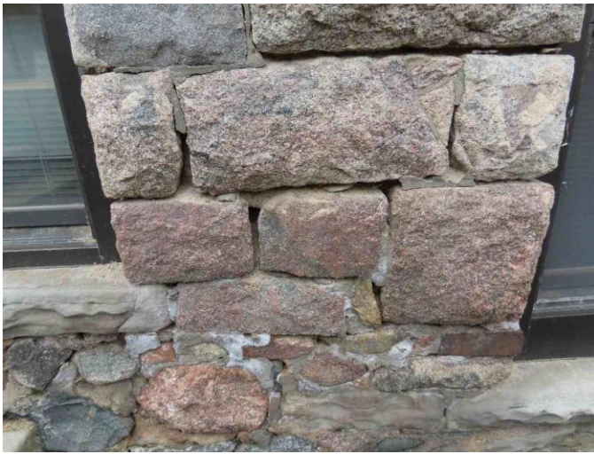
North Elevation Granite Foundation Walls — The coursed granite base is in fair condition with many large voids in the mortar joints.
