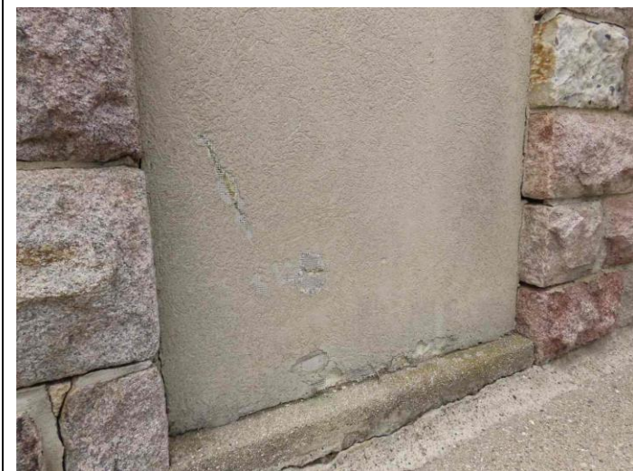
EIFS Infill Damage
