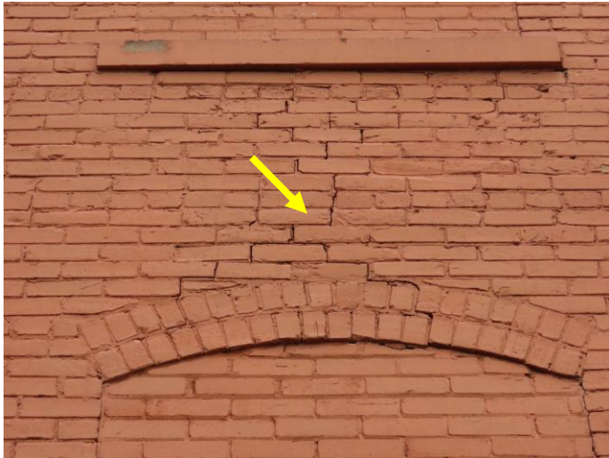
Masonry Cracking, Typical
