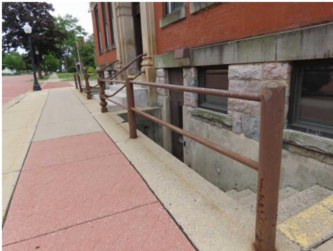
North Elevation Steel Railings — Steel railings are heavily corroded. They should be thoroughly cleaned and coated, and perhaps removed and sandblasted to arrest the damaging corrosion.
