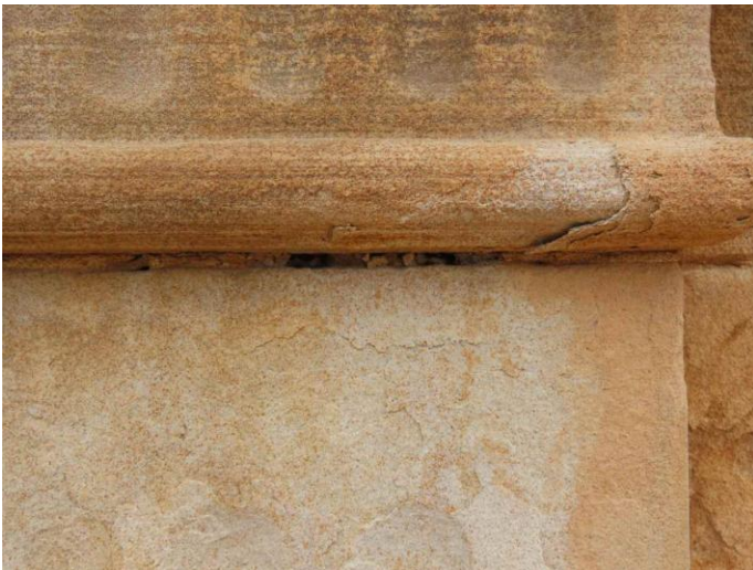
North Elevation Front Entry – Detail of deteriorating sandstone molding, typical.
