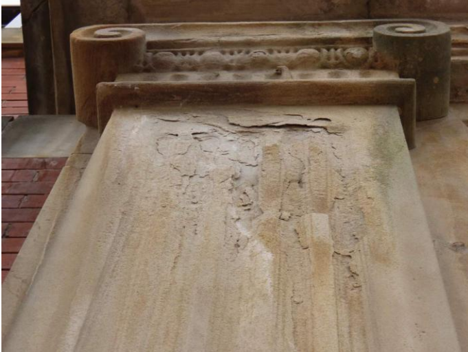
North Elevation Front Entry – Detail of deteriorating sandstone pilaster.
